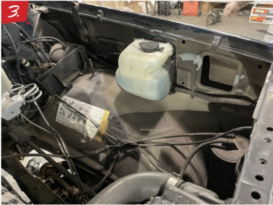
3. Harrison starts with the driver side inner fender. There isn't a whole lot to remove here. The factory bottle jack is missing like most of these trucks, but we will need to address the vapor canister mount.
